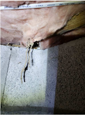
Termite shelter tubes in the crawlspace
