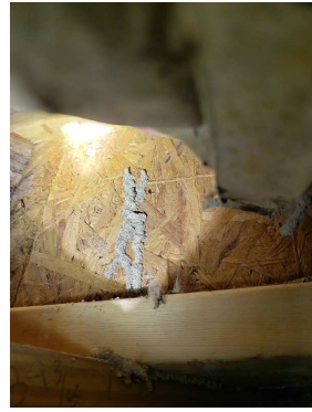
Termite shelter tubes in the crawlspace
